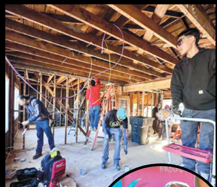
In San Diego, EWMC members from Local 569 headed to the neighborhood of Southcrest, where they installed new electrical wiring, devices, and upgraded the subpanel for a family who hadn't been able to move back into their home since flooding in January of 2024. Inset are journeyman wiremen Billie Johnson, left, and David Johnson, no relation.
